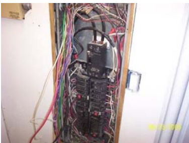
Existing 200A Electric Service Switch
